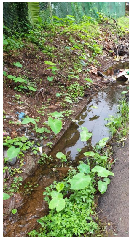
Fig No. 4 Poor Drainage Design (
